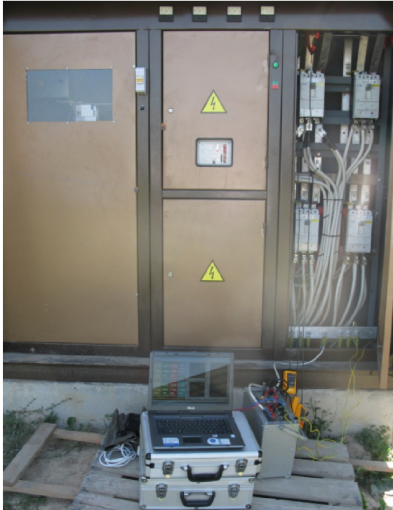
Fig. 2. Connection of portable quality analyzer to the bus of 0.38 kV transformer substation FES
