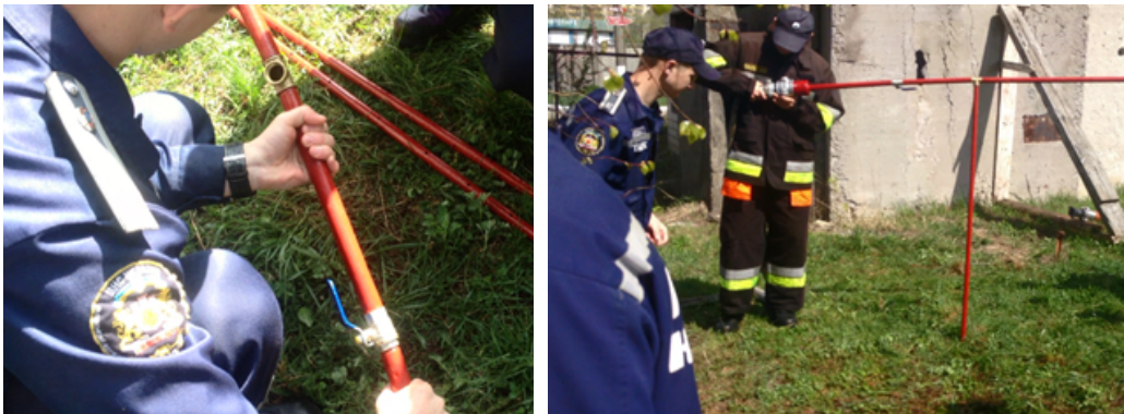
Figure 19. Drafting and installation of a developed peat fire extinguishing system
