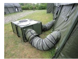
c) mobile air conditioning system
